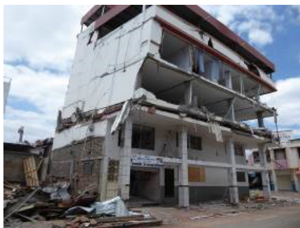
Figure 3: Weak/soft storey failure
