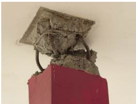
Figure 2: Inadequate design and detailing for shear link spacing and detailing
